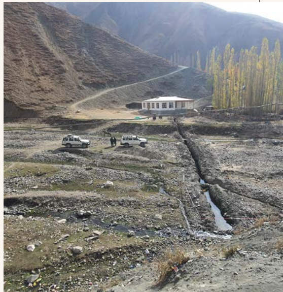
LEFT: Community members participate in the construction of water infrastructure, ensuring a sense of local ownership.
